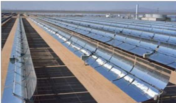
Figure 6. Parabolic Collector of the Power Plant.
